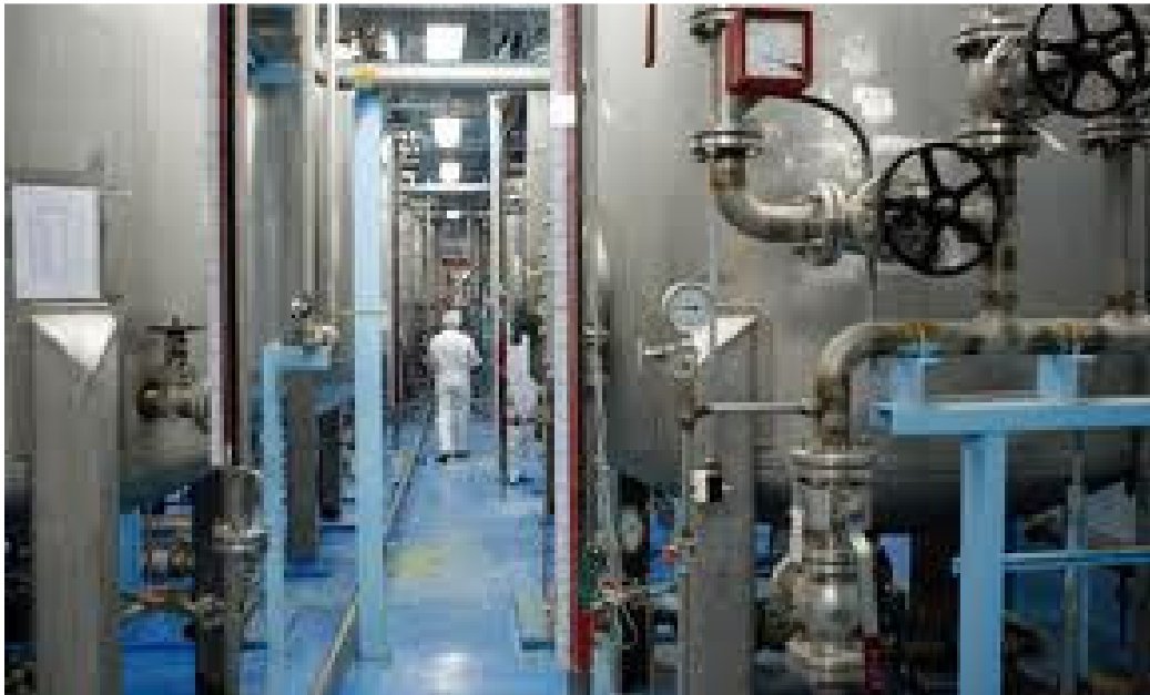
Figure 11. Iran's uranium conversion facility at Esfahan. Photo: Photograph: Caren Firouz/Reuters 129
